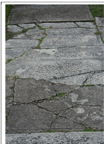
Footpath in poor condition (8 to 9 rating).
