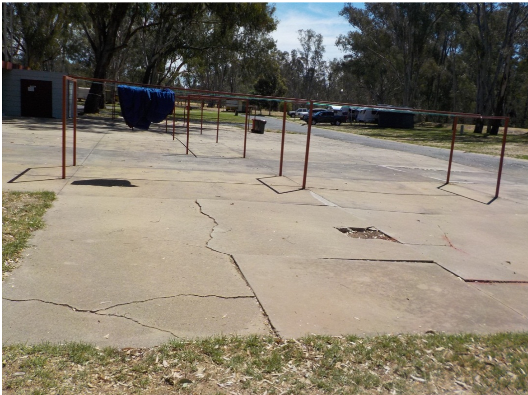
Various trip hazards and poorly designed cloths line which pose significant OHS issues to visitors
