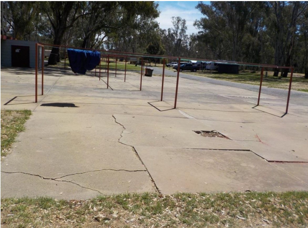
Various trip hazards and poorly designed cloths line which pose significant OHS issues to visitors
