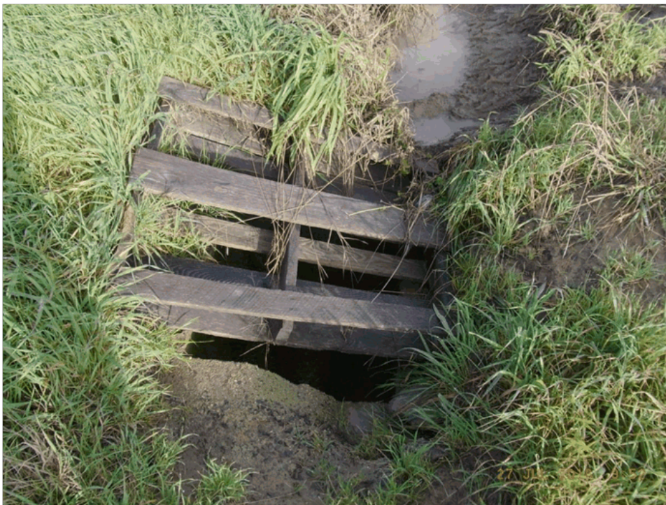
Drainage pit at the proposed vehicle crossing to the child care centre site
