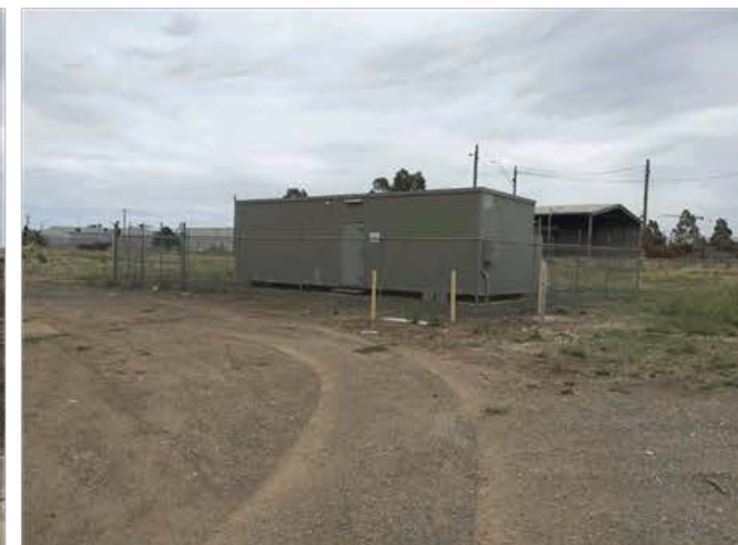
Figure 15 Building No.20 High security fenced and windowless electrical substation off Purcell Street (for supplying V/Line signaling power)
