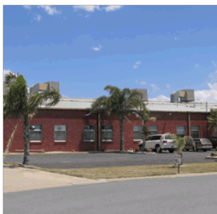
Avoid: Visible plant and building services on roofs that are not screened from the public realm
