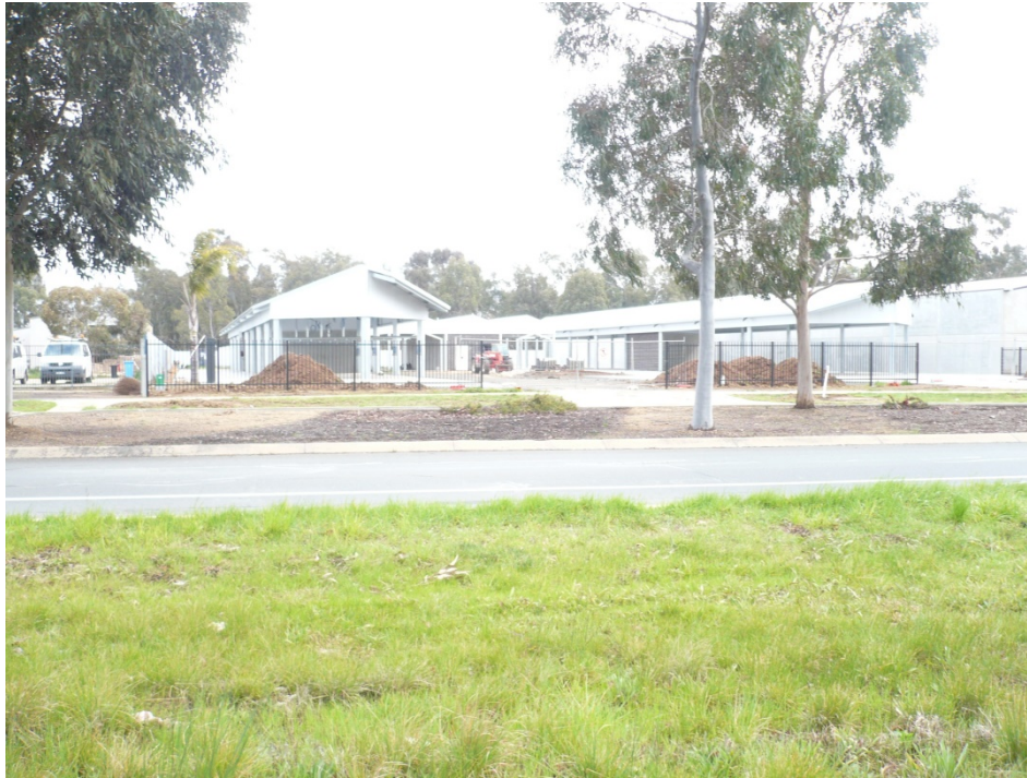
Car wash at the western end of the land which is under construction
