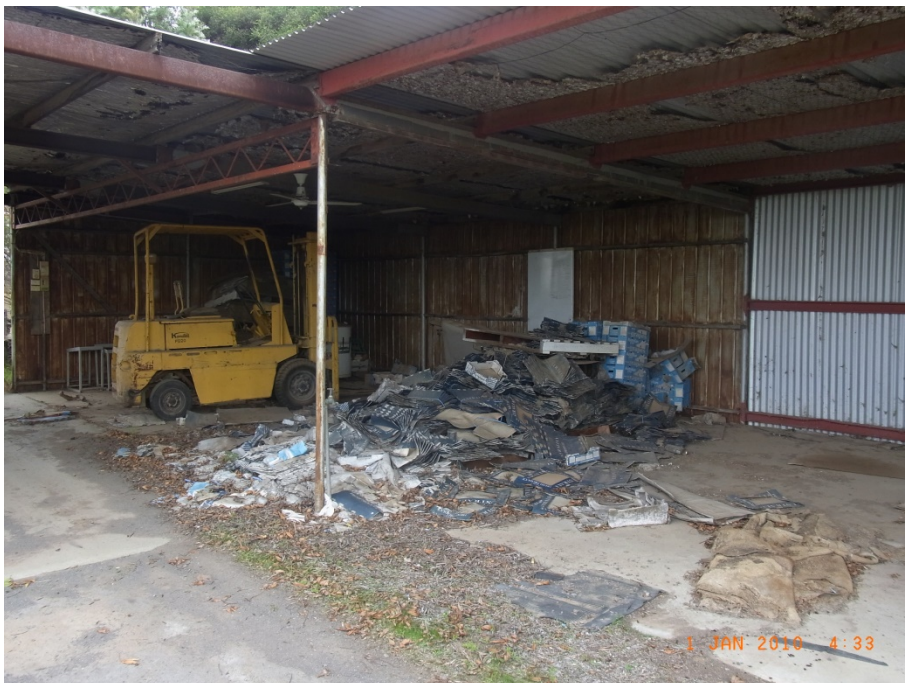
Looking south into packing shed where grading and packing previously took place
