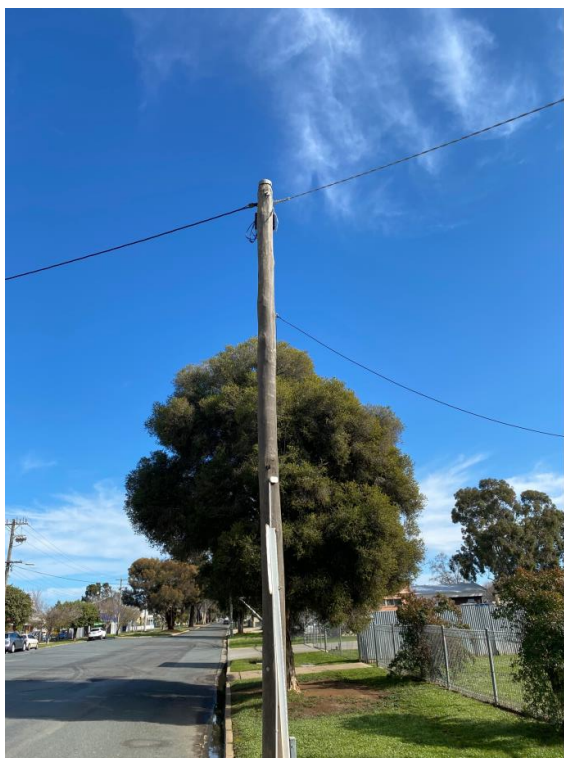
Existing power pole in Casey Street nature strip which provides overhead connection to a dwelling that is to be demolished.
