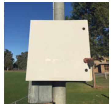
Irrigation cabinet example
